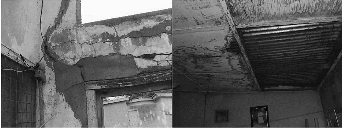
Figure 4: Faded painting, cracked walls and rotten ceiling of some public housing units
